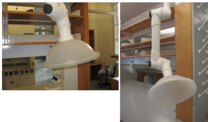
Figure 9. Two images of snorkel ducts in labs.
