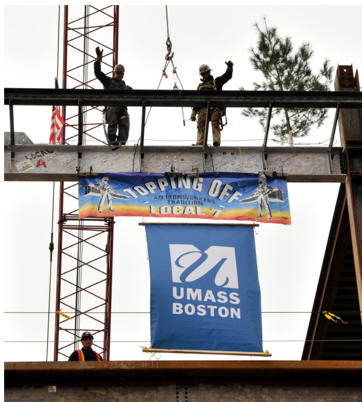
Ironworkers prepare to place a steel beam signed by UMass Boston community members, complete with a seedling tree to represent growth and good luck, atop the frame of the Integrated Sciences Complex. UMass Boston hosted a program of speakers for the topping-off ceremony on February 16.
